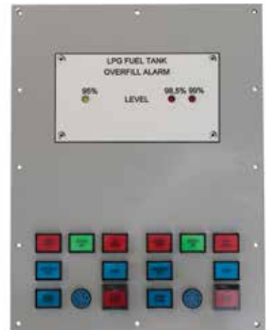
Panel with alarm overview on each tank
