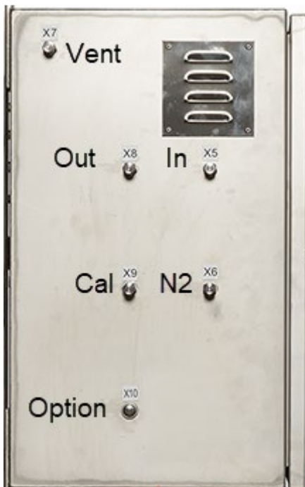
Figure 8 Analyser cabinet, left side view
