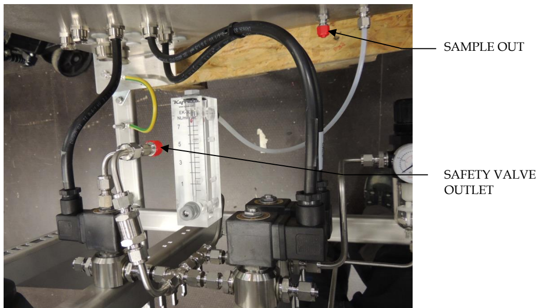
Figure 38 Plugs under analyser cabinet to be removed before start-up
