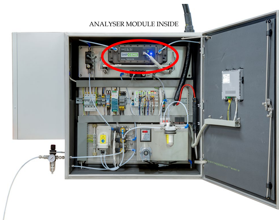
Figure 6 Analyser cabinet, interior view
