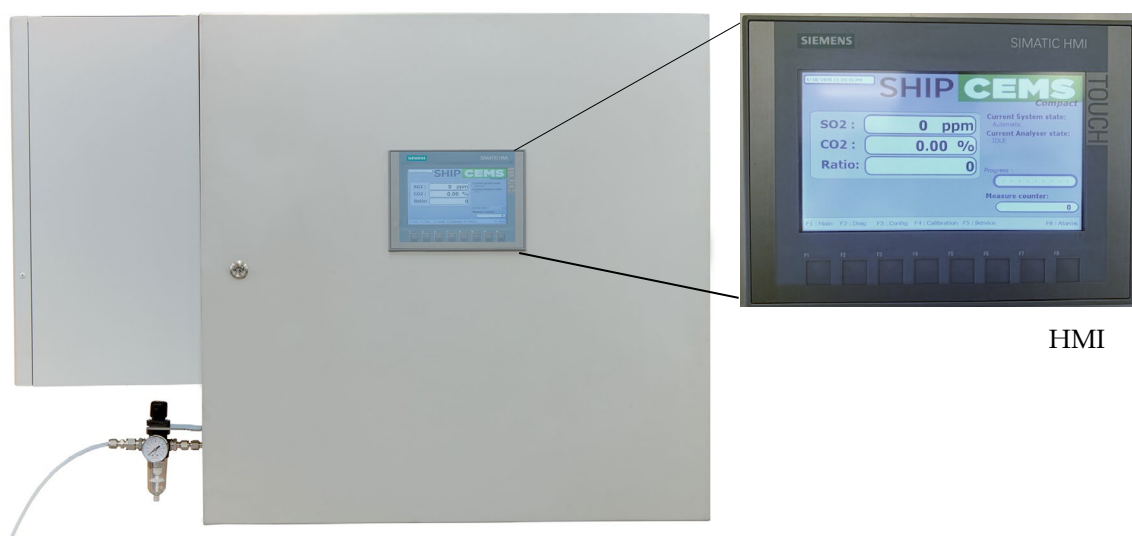
Figure 4 HMI in front of the analyser cabinet
