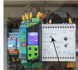
MOISTURE SENSOR ALARM INDICATOR
