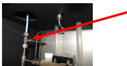
Figure 7 T-piece in the SCS cabinet
