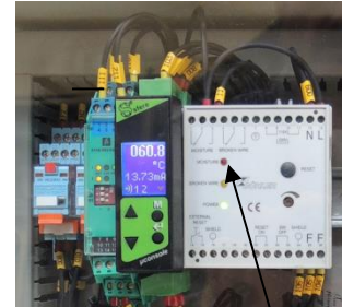
MOISTURE SENSOR ALARM INDICATOR
