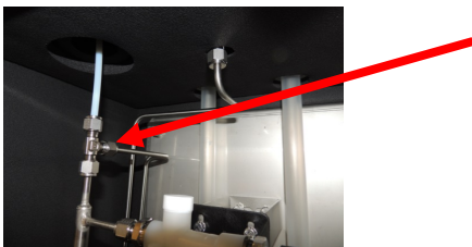
Figure 7 T-piece in the SCS cabinet
